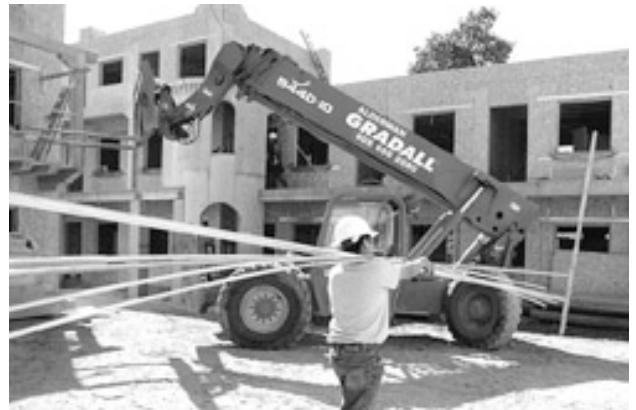
Montecito Bank & Trust has committed $500,000 to the Housing Trust Fund of Santa Barbara County, which helps facilitate affordable housing projects in the area, such as the 62-unit El Carrillo apartment complex in Santa Barbara, at top. STEVE MALONE/NEWS-PRESS
